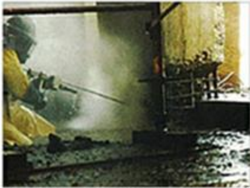
Concrete Pillar Breaking
